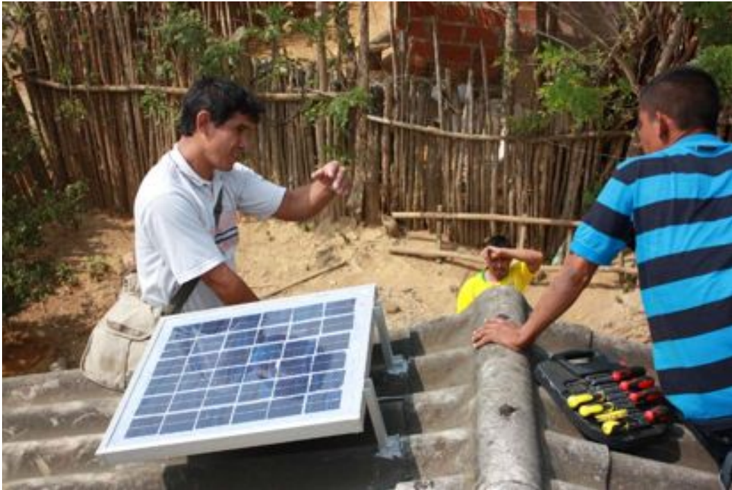
Installing a 32 watt PV module on a home in the Juaruco village
