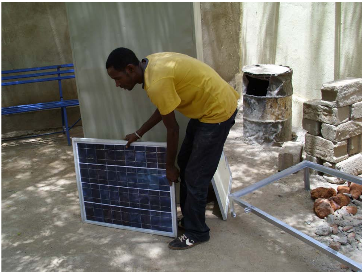
Preparing the two 60 watt PV modules for installation on the women's birthing center.
