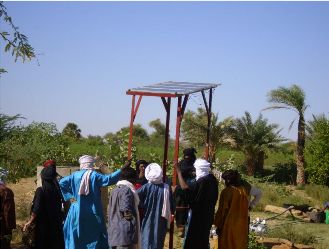
Erecting the tower with the PV modules to power the solar water pump for the well in the background.
